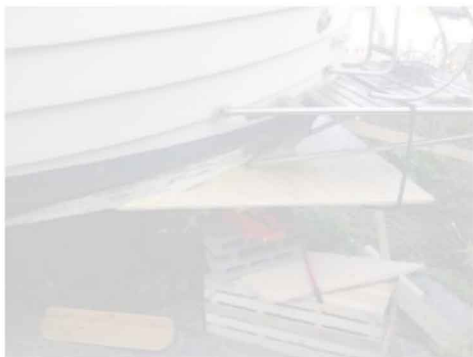
The flap was held in place with jacks while the epoxy set
